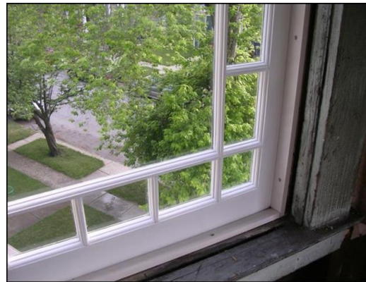
The same window before and after restoration; Courtesy of Steve Swiat, Northwood Restoration, Buffalo
